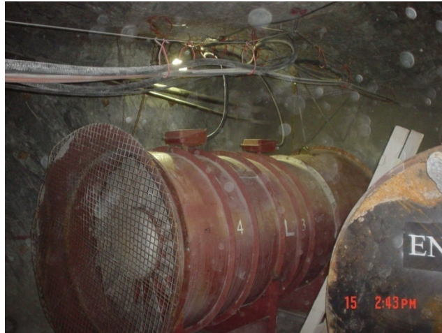
Figure 7 - 900m level booster fans
